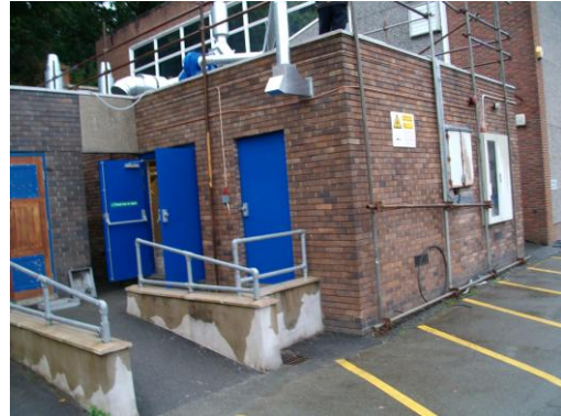
External bulk Chemical Store
