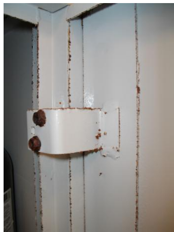
Signs of corrosion
